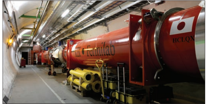
Inner triplet assemblies positioned in the LHC tunnel in 2006.
