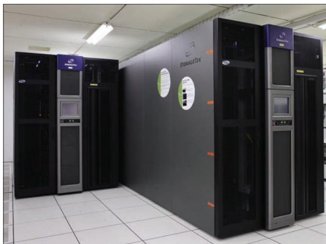
Part of the CASTOR mass-data storage system at CERN.
